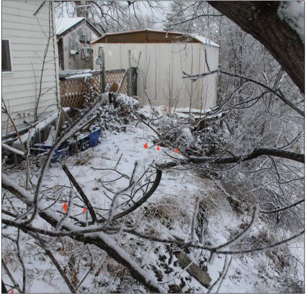
Undermined Deck and Telltale Flags – 239 Houston Ave
